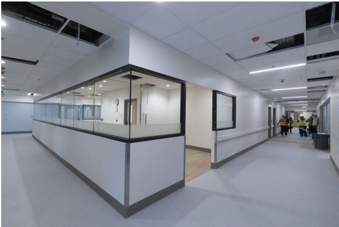
1 of 5 | The University of Washington Center for Behavioral Health and Learning at the UW Medical Center's Northwest campus is expected to be ready for occupancy next year. (Ellen M. Banner / The Seattle Times)
